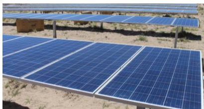
Invenergy developed project, Luning Solar Energy Center, located in Luning, Nevada
